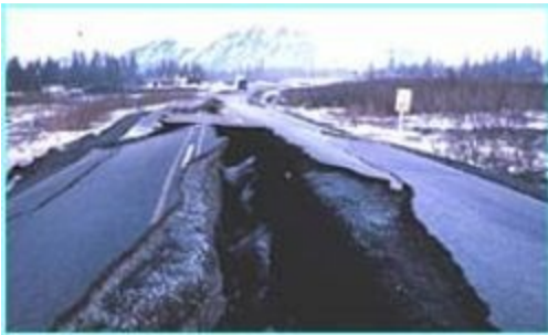
An Alaskan earthquake caused the ground to crack apart.
