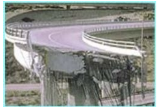
This highway in California collapsed during an earthquake.
